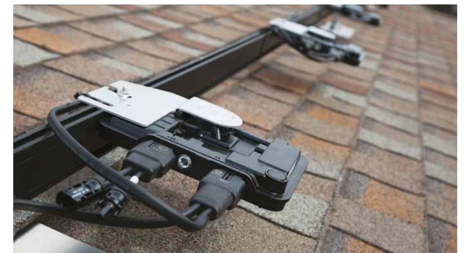
IQ microinverters in a rooftop installation
