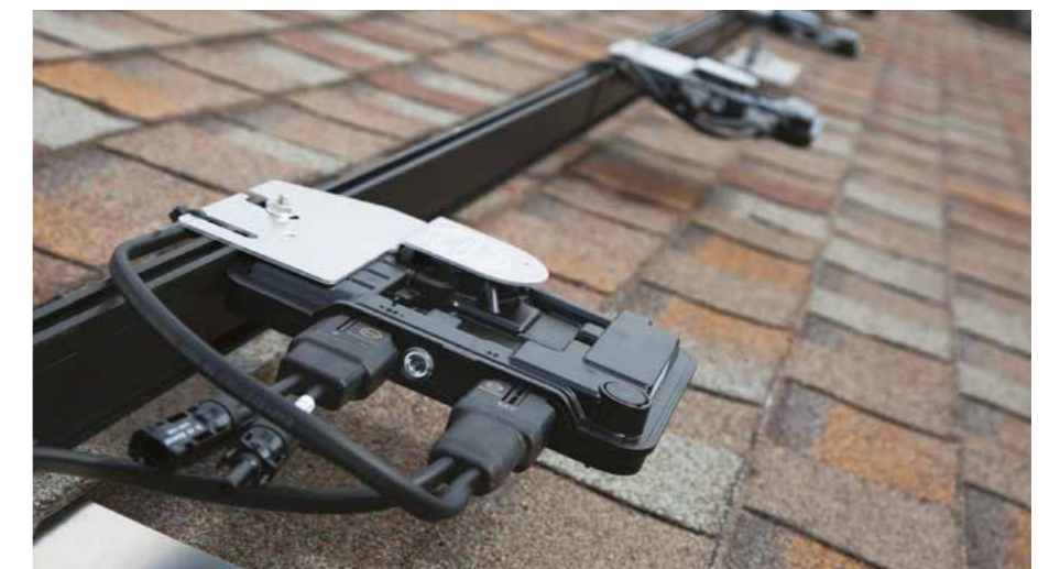
IQ microinverters in a rooftop installation
