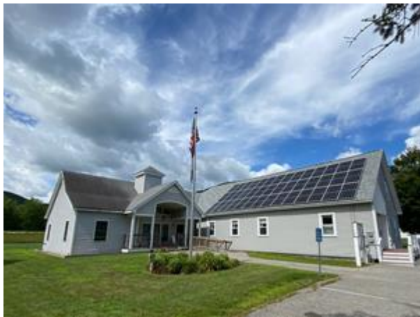
Enphase Energy and 603 Solar to Offset 100% of Energy for Shelburne, NH Town Hall
