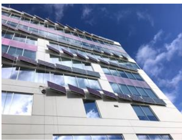
MoZaic East (by Ackerberg Group) is a building-integrated photovoltaic (BIPB) commercial solar project in Minneapolis, MN. Solar design and installation: All Energy Solar; inverter technology" Enphase Energy; solar module overlays: SolarSkin from Sistine Solar
