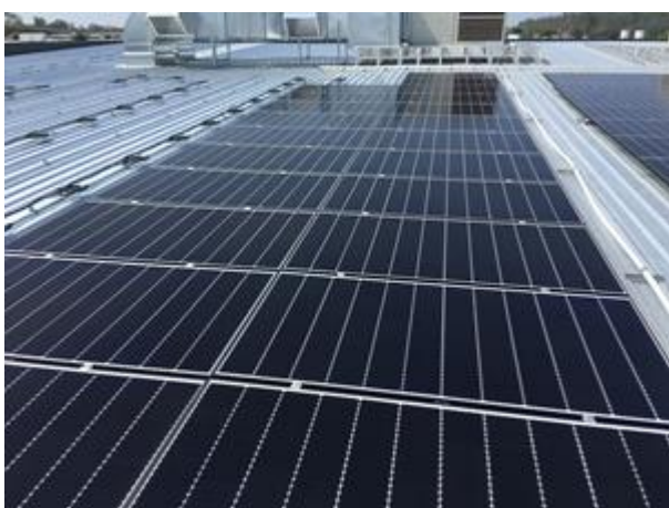
REA deployed an 80 kW solar system pairing its Power Series modules with Enphase microinverters for Innovative Stainless Steel in Brisbane, Queensland.
