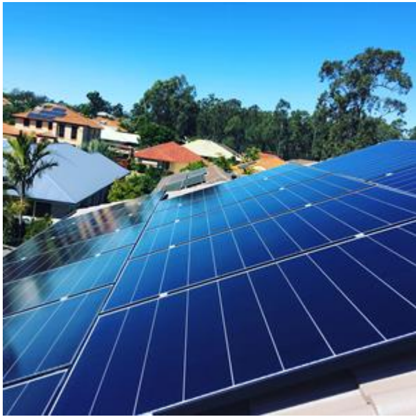
Enphase microinverters enable REA to install panel arrays across multiple roof areas and orientations to maximize solar power production.
