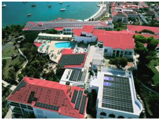
The commercial solar system installed by ProSolar Systems at Bluebeard's Castle Resort in the Caribbean, featuring Enphase microinverters.
